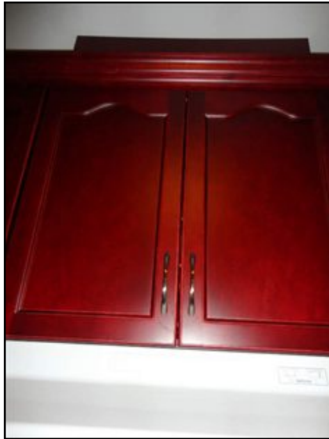
27. Gap between cabinets and ceilings or walls
