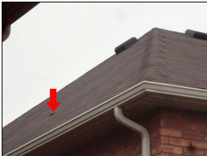
6. Asphalt shingles not sealed
