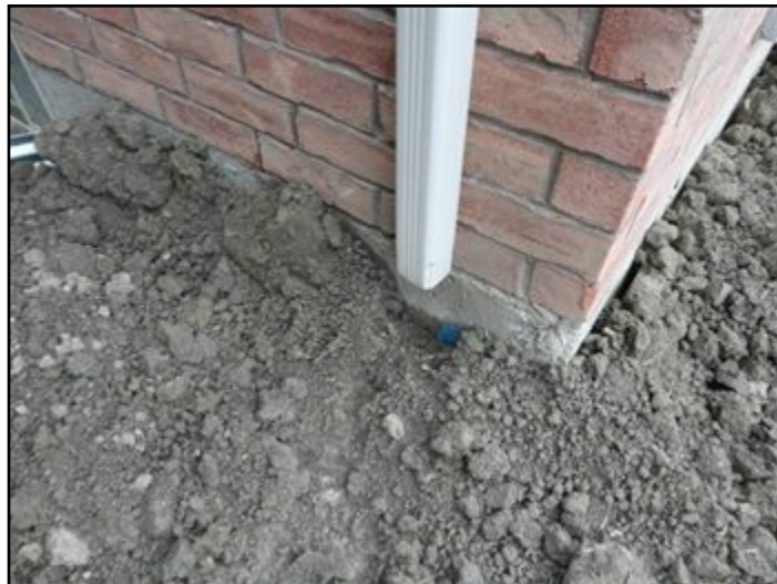
43. Missing splash blocks/rainwater leaders
