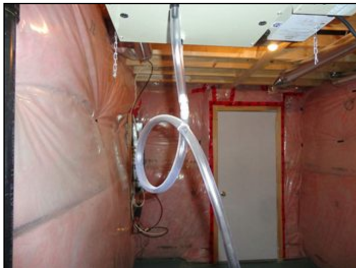
16. Condensate line is blocked
