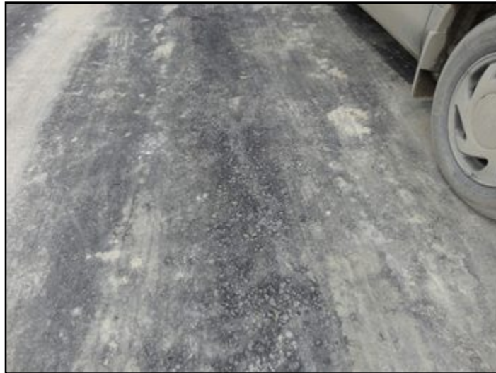
42. Driveway has settled
