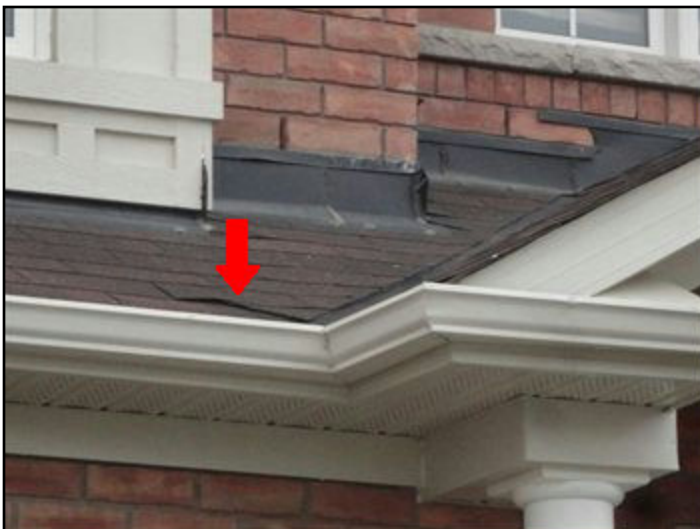
5. Asphalt shingles not sealed
