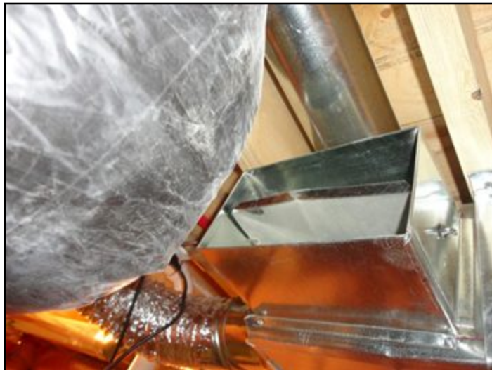
22. Heating, ventilating or air conditioning...
