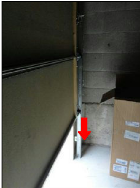
35. Garage doors do not operate properly
