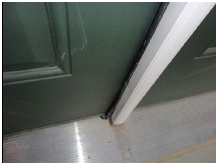
21. Air infiltration through windows and doors
