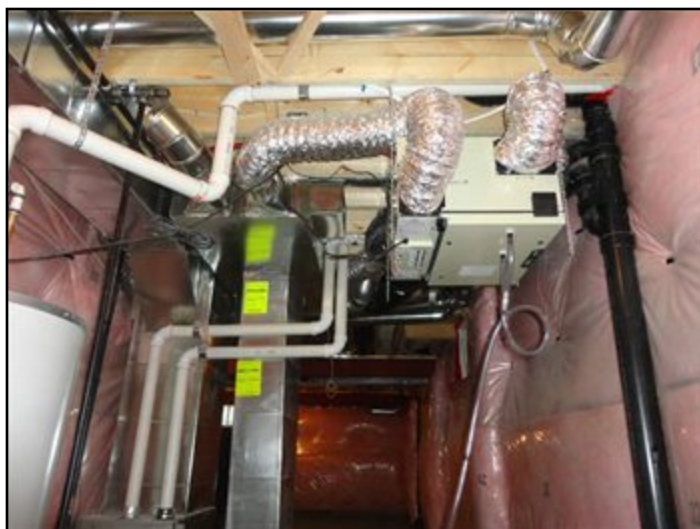
23. Heating, ventilating or air conditioning...
