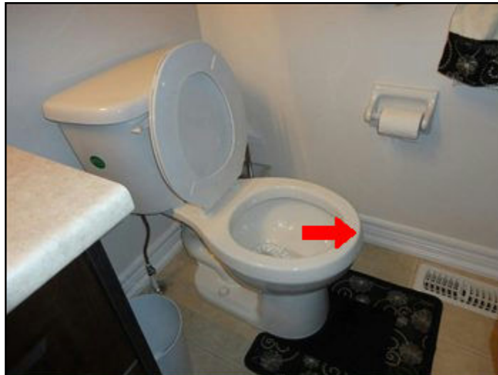
9. Defective plumbing fixtures, appliances or...
