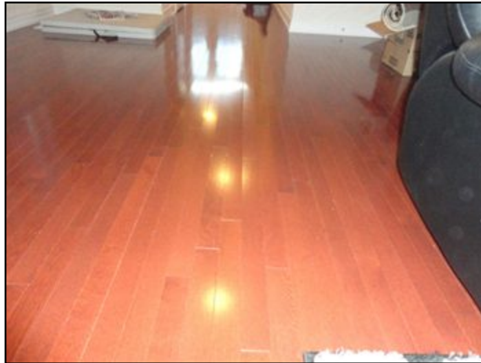
29. Floor is uneven
