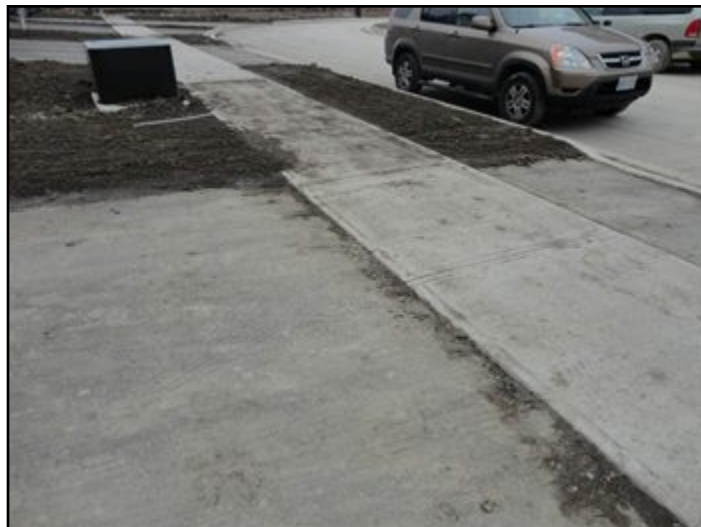
37. Water ponding in surface grading of the site
