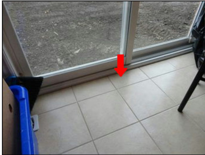
20. Air infiltration through windows and doors
