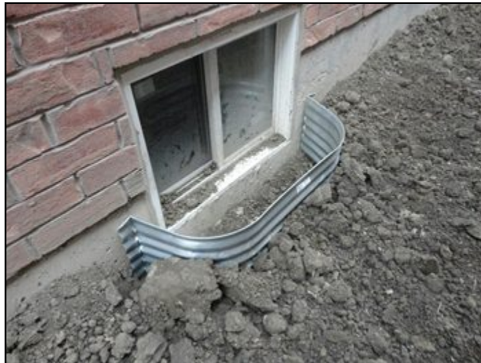
38. Water ponding in surface grading of the site
