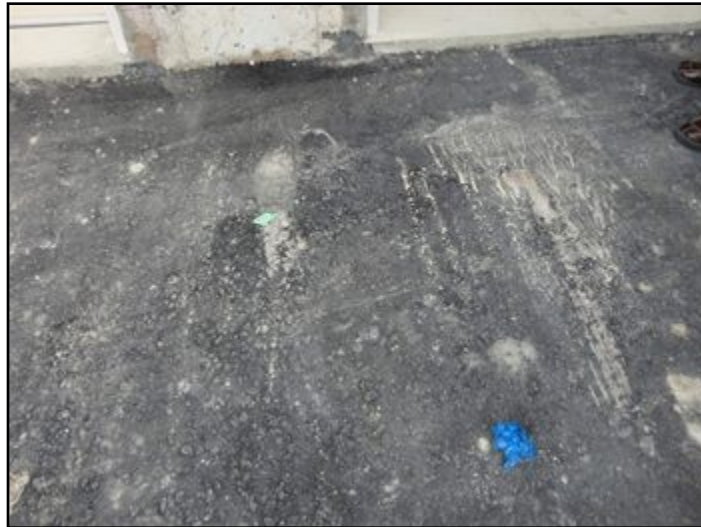
36. Driveway has settled
