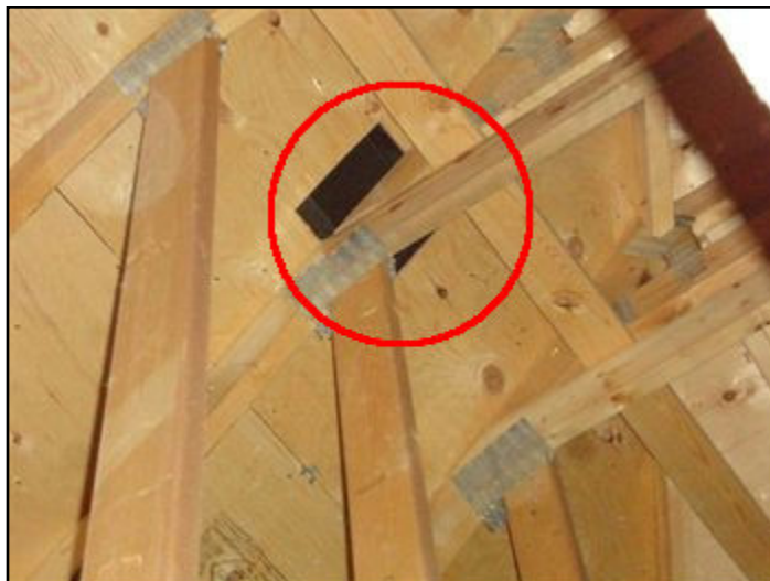
4. Inadequate attic ventilation
